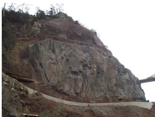
Fig. 13 – Area that suffered a landslide.
